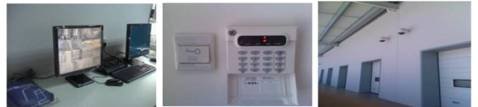
Security system: CCTV systems, infrared alarm systems, electronic access control system
